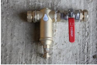
Spirotrap fitted with a single full-flow lever valve (25 Kw Unit).
